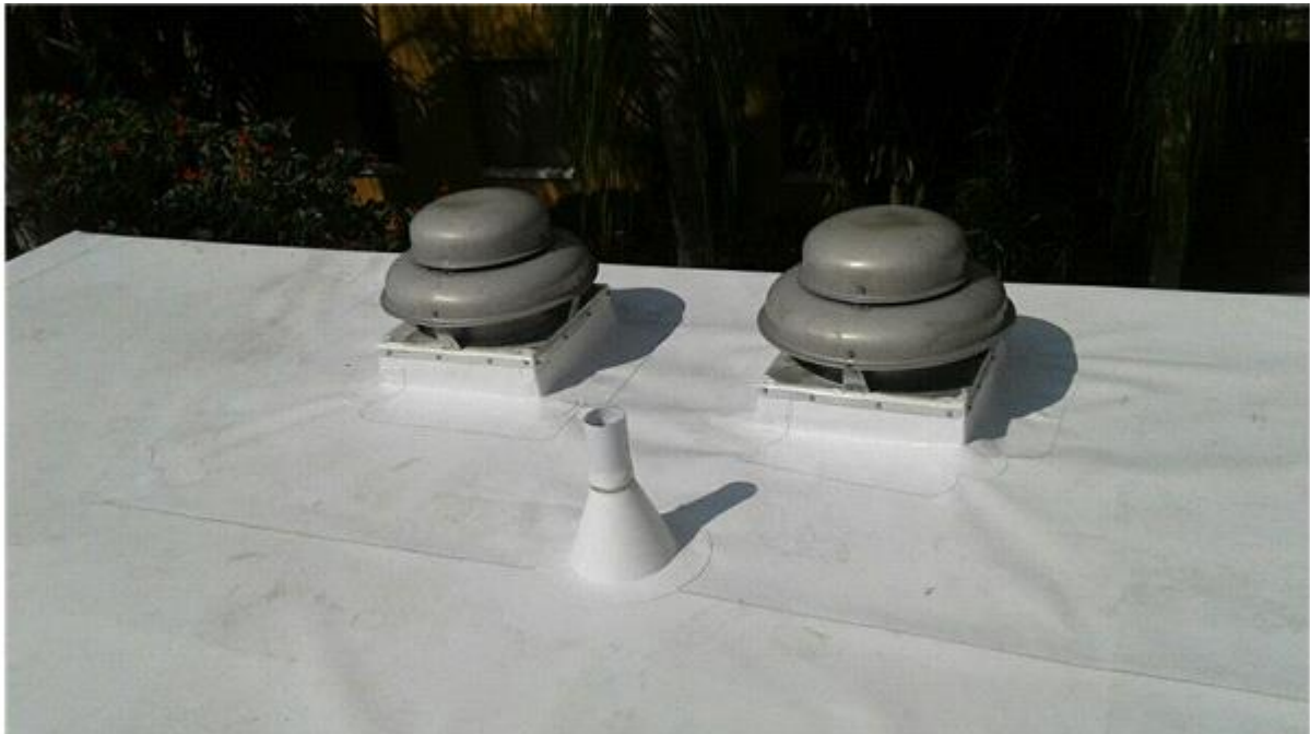
004G -Base Flashings The base flashings appear to be in good condition.
