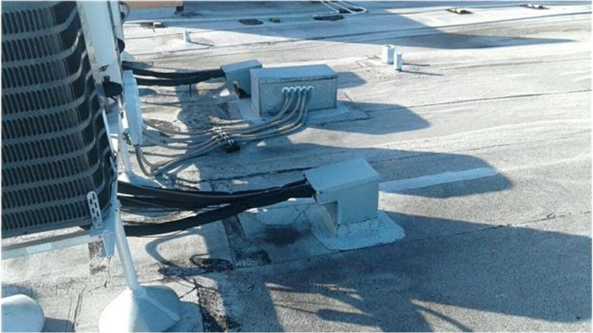
010F- Equipment Housing
