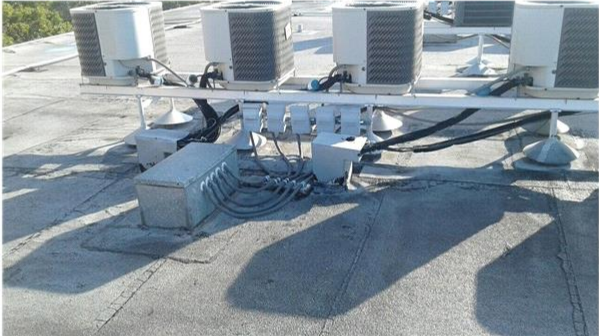
010F- Equipment Housing
