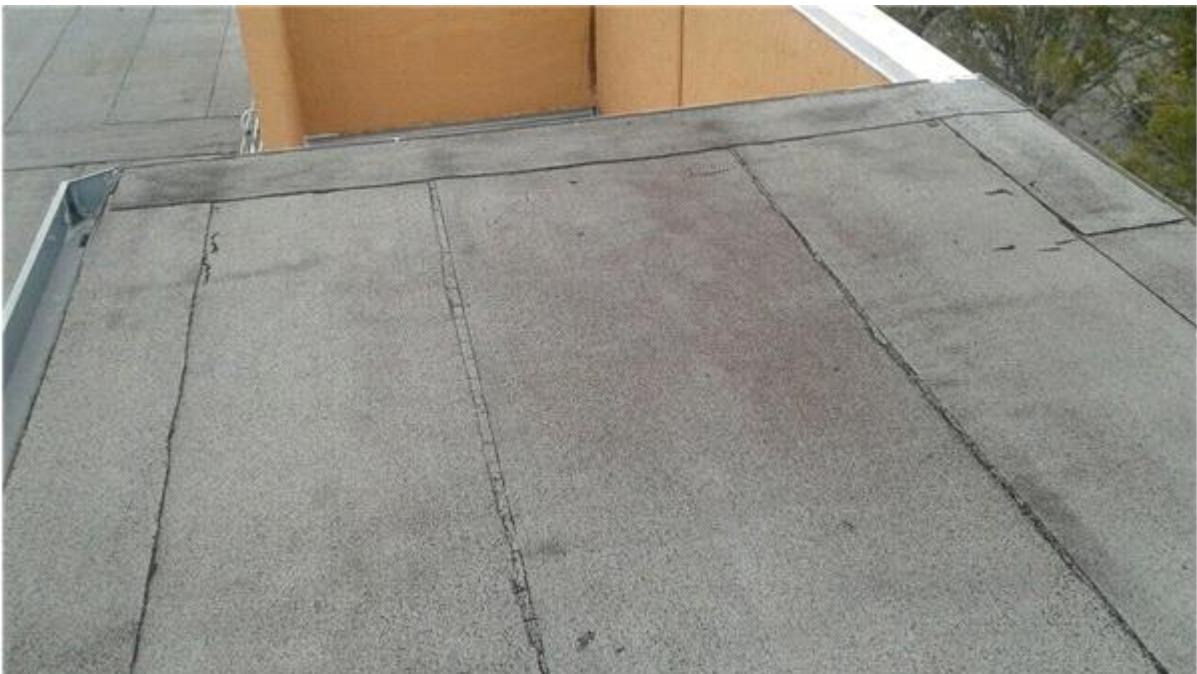
003F -Membrane Overview The roof membrane appears to be in fair condition at this time.
