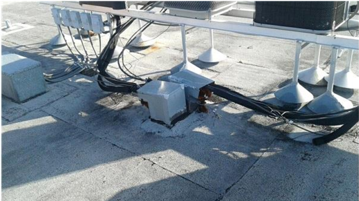
010F- Equipment Housing
