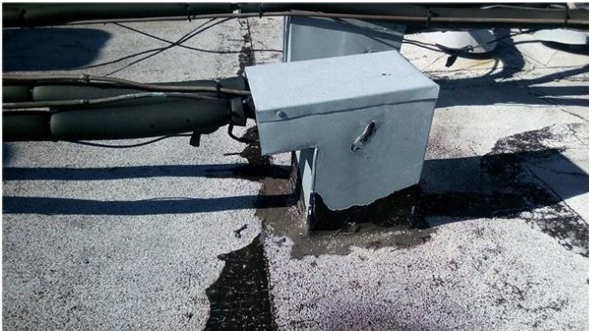
010G- Equipment Housing
