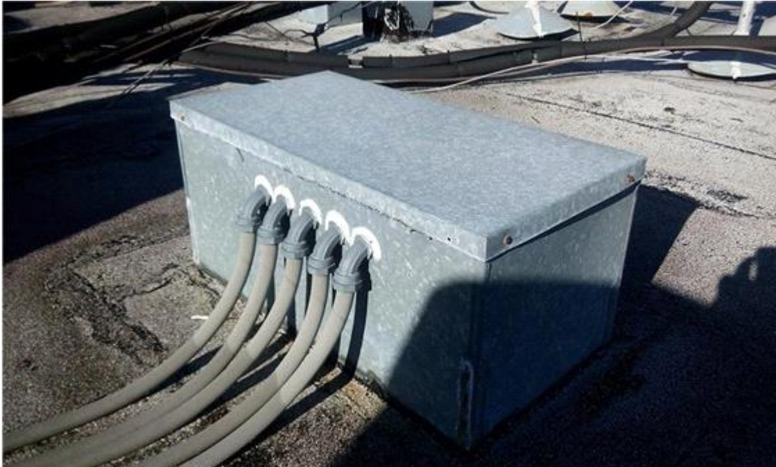
010G- Equipment Housing
