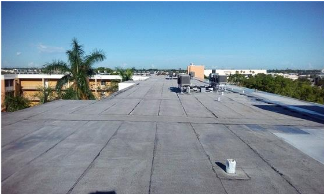
001F - Surface Overview The roof surface appears to be in fair condition at this time.
