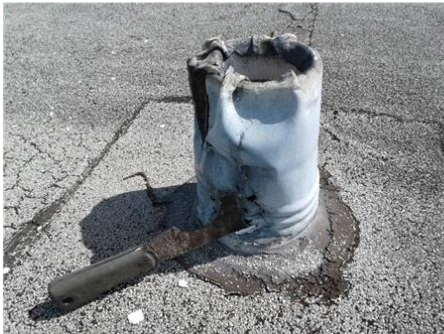
Damaged Lead Boot
