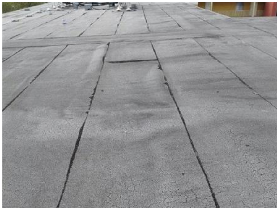
F-202 Field Membrane Blister
