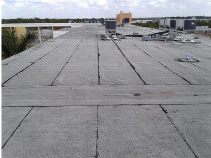
F-202 Field Membrane Blisters
