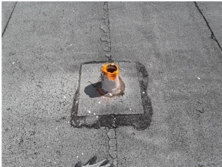
Damaged Lead Boot
