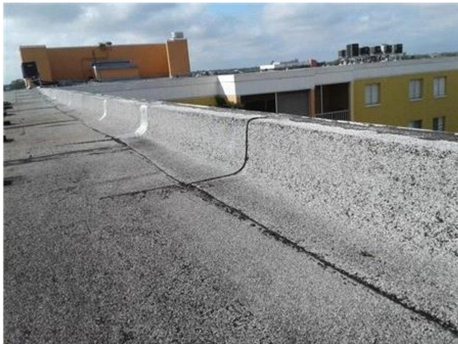
004G - Base Flashings The base flashings appear to be in good condition.
