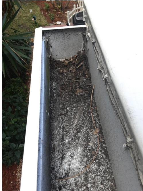
Debris in Gutter
