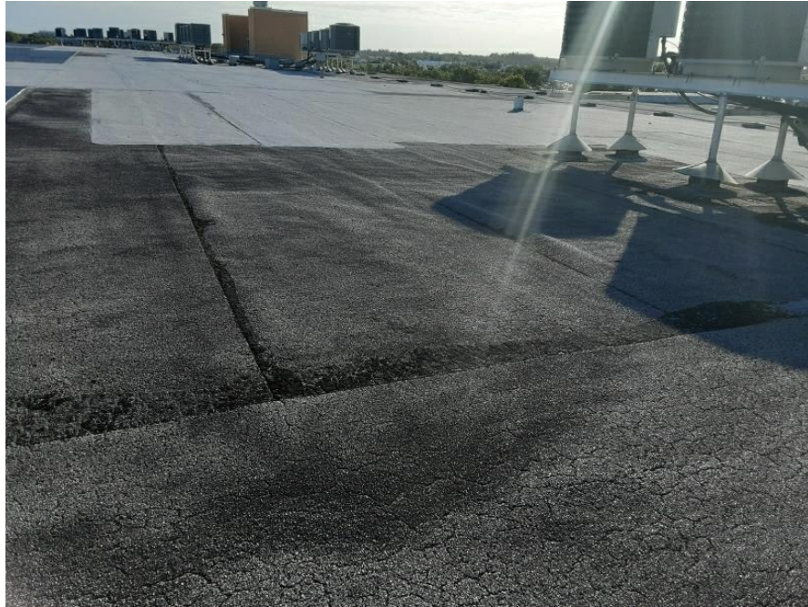
Field Membrane Blister
