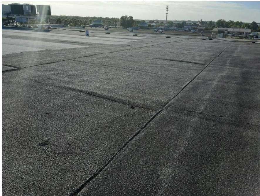
Field Membrane Blister
