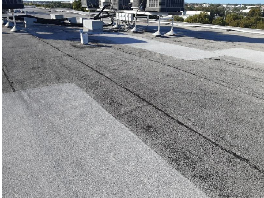
Field Membrane Blister
