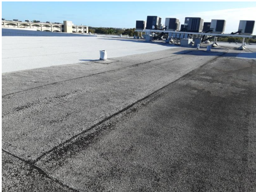
Field Membrane Blister
