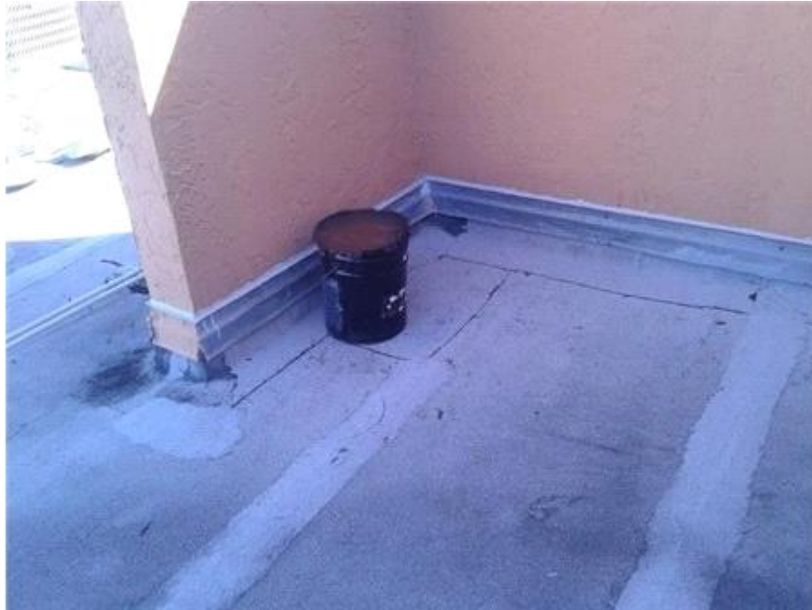
Stairwell Roof: Debris on Roof
