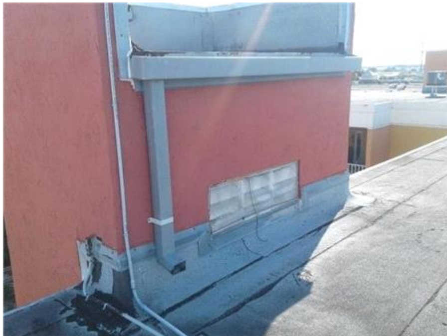
Elevator Shaft Roof: Appearance Overview The appearance of the roof is in fair condition at this time.
