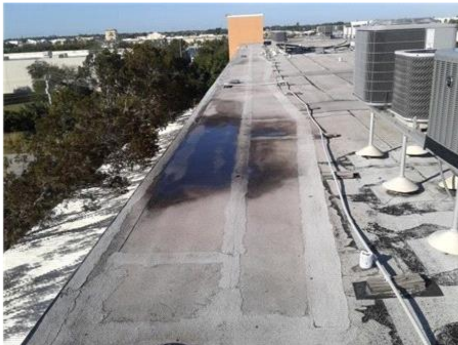
Main Roof: Ponding
