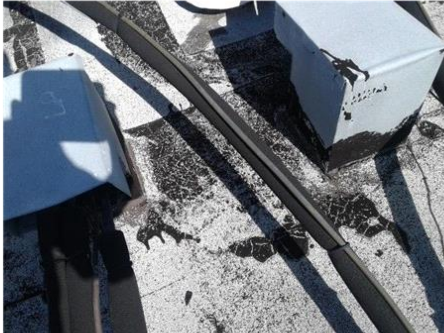
Elevator Shaft Roof: Sealant Deterioration/Failure
